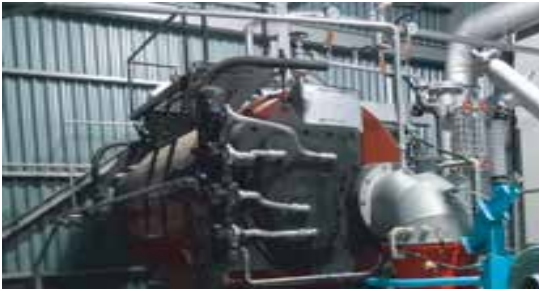
1ton small boiler
