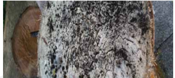
Rapid decay due to moisture and glucose
