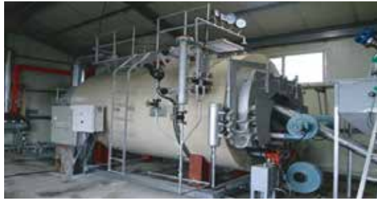
5ton steam boiler
